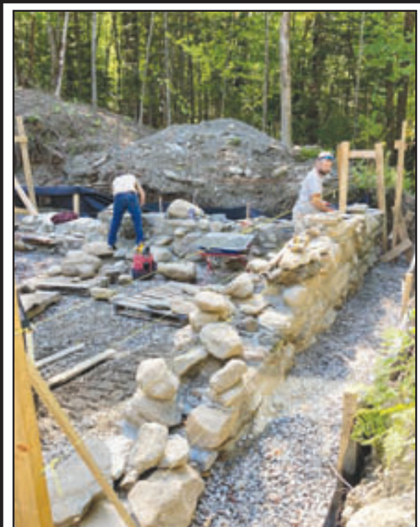
Stevensville Cabin update: just a quick note to say that the foundation is coming along well. If the weather holds, it will hopefully be complete in the next few weeks. Feel free to go check it out if you are in the area! Also, if you are interested in supporting the project financially, you can do so at: www.stevensville-cabin.org . All contributions are greatly appreciated. PHOTO CONTRIBUTED
